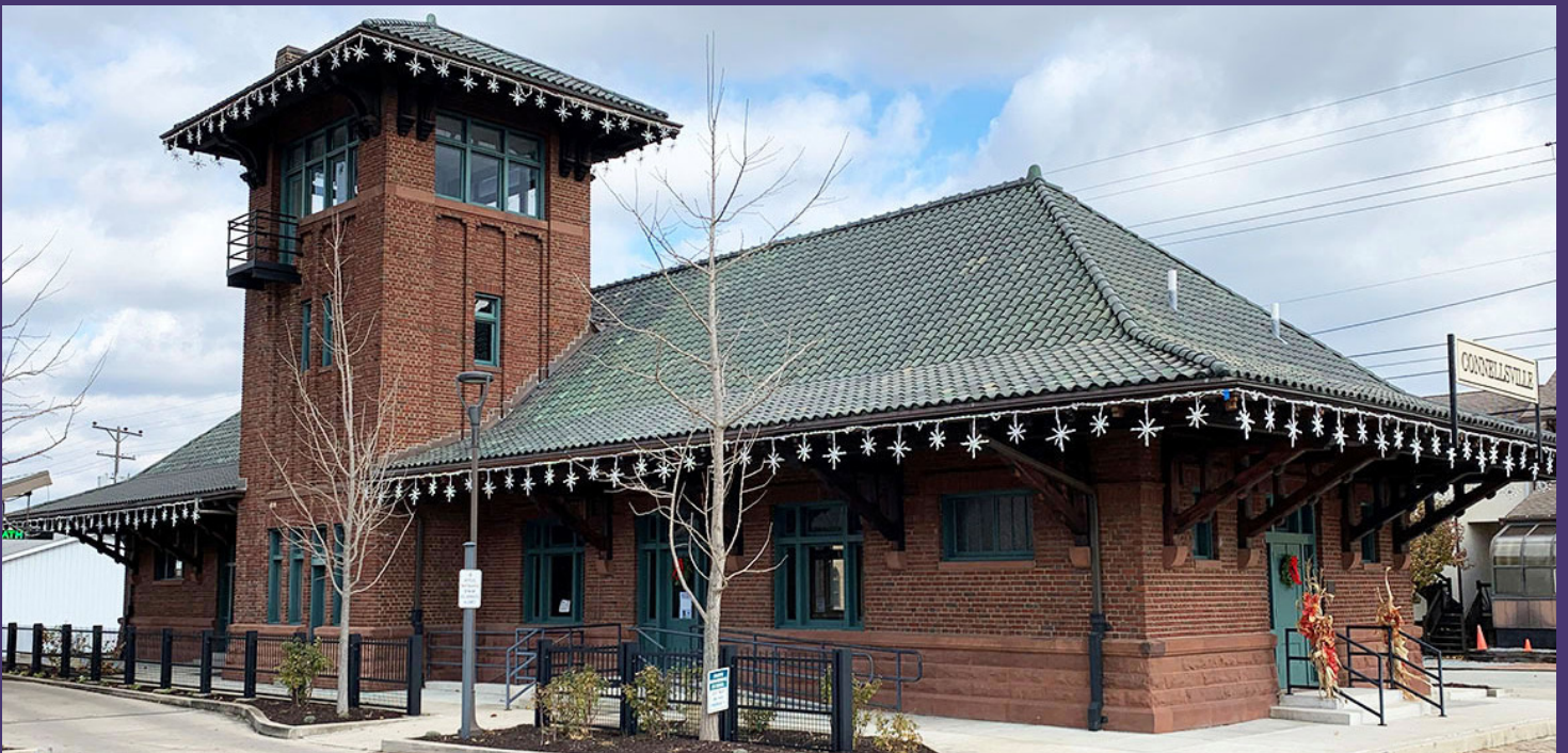
Rehabilitation work on the exterior included repair of historic masonry, windows, decorative wood details, lighting, and the roof and the installation of new doors and ADA access. The work preserved the building's distinctive tower, roofline, and overall character.
