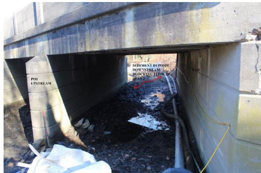
Photo 20 Pump discharge pipe in Span 2
