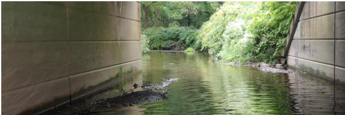
Photo 46 Sediments Built-up and Debris in Downstream of Span 2
