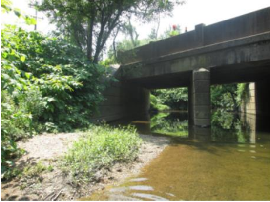
Photo 1 Span 2 Looking Upstream Sediment Deposition
