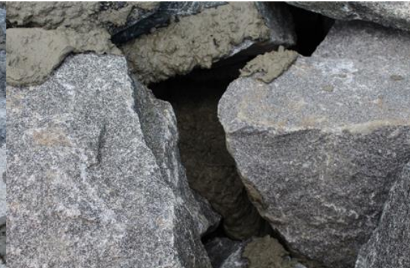
Photo 10 Grout Fell to the Bottom of the Voids
