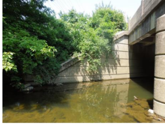
Photo 2 Span 1 Looking Down Stream Formation of Scour Hole
