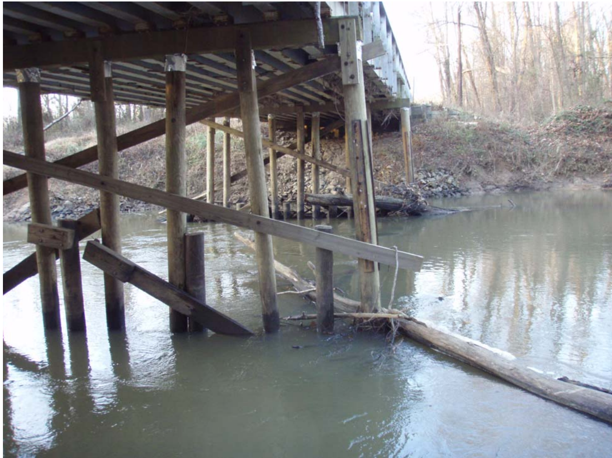
Figure 4. Crib structures could be installed on the exposed multiple piles supporting this bridge to prevent debris from becoming trapped between the piles.
