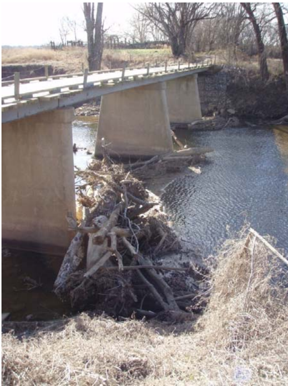
Figure 24. VA 603 bridge over a branch of the James River, Goochland Co., VA.
