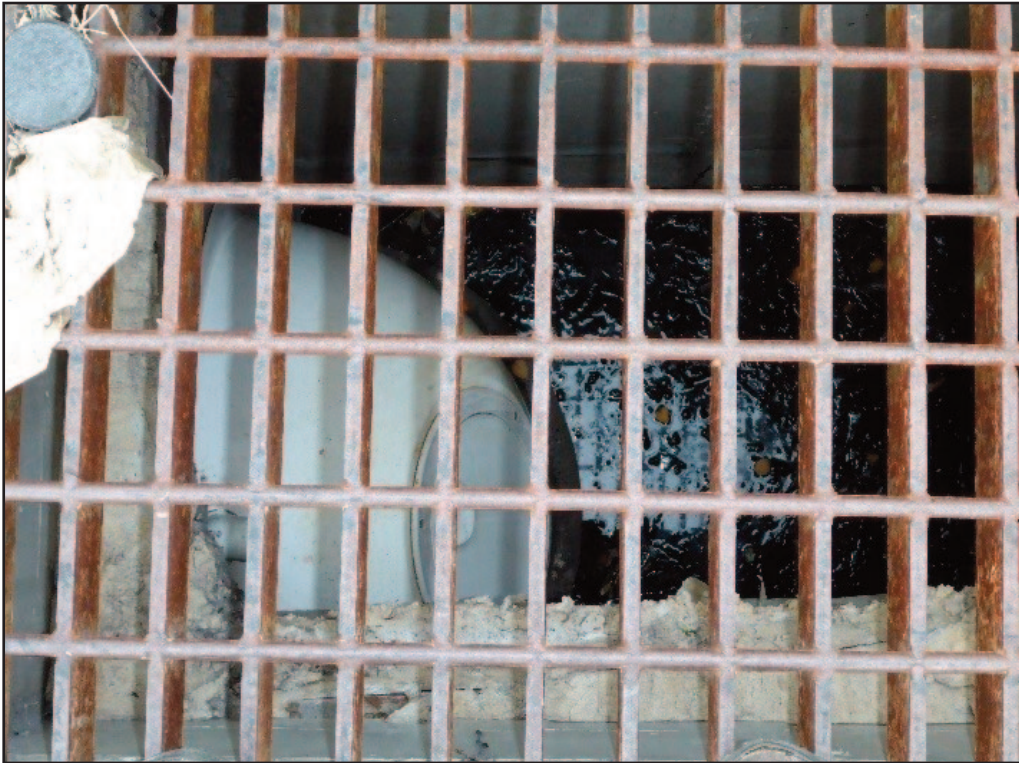
Figure 6.4.1: Inlet with Sump/Trap (photo c/o: Pennsylvania Turnpike)
