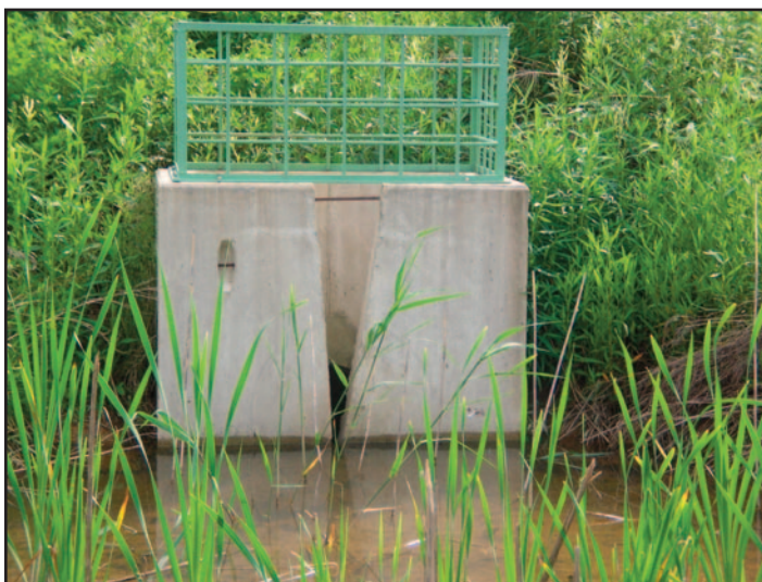
V-notch weir with top mounted trash rack
