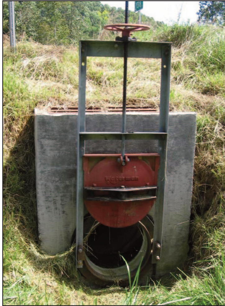
Figure 5.2.4: Open Screw-Type Sluice Gate (c/o NCDot-HSP-2010-01)
