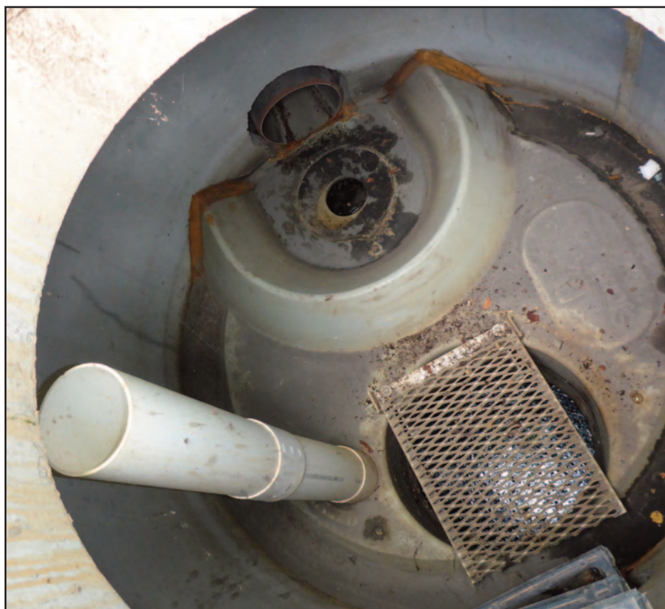
Figure 5.13.1: Manufactured Treatment Device – Hydrodynamic Separator
