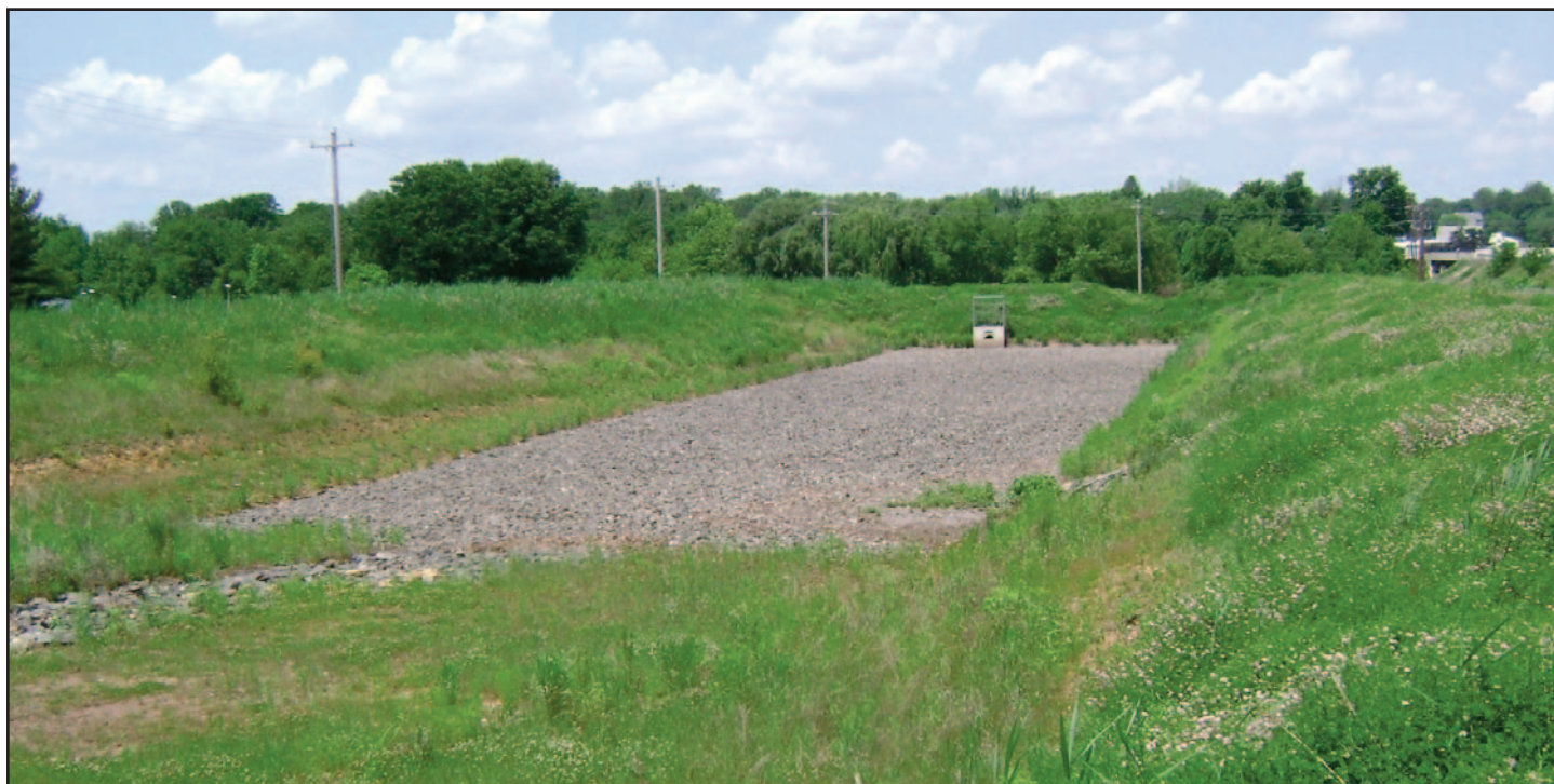
Figure 5.3.1: Infiltration Detention Basin with Engineered Soil Surface
