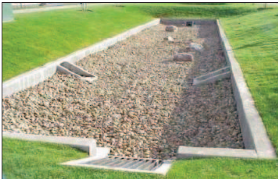
Figure 5.8.1: Open Constructed Stormwater Filter (photo c/o PADEP BMP Manual 2006)
