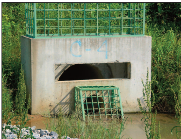
Rectangular weir & circular orifice with trash racks
