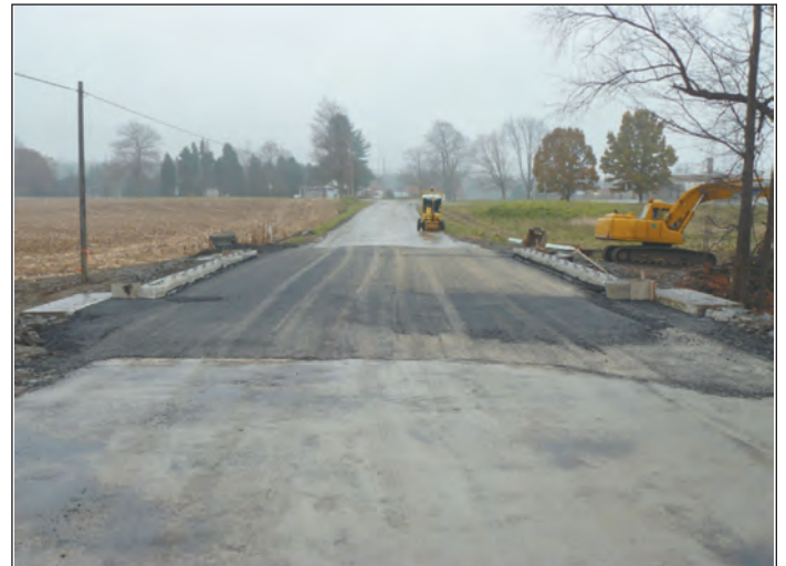
Placement of barriers and bituminous overlay (non-composite), backfill, paving, and installation of traffic safety features by Department Forces.
