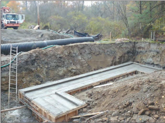
Removal of existing bridge and installation of cast-in-place spread footing by Department Forces
