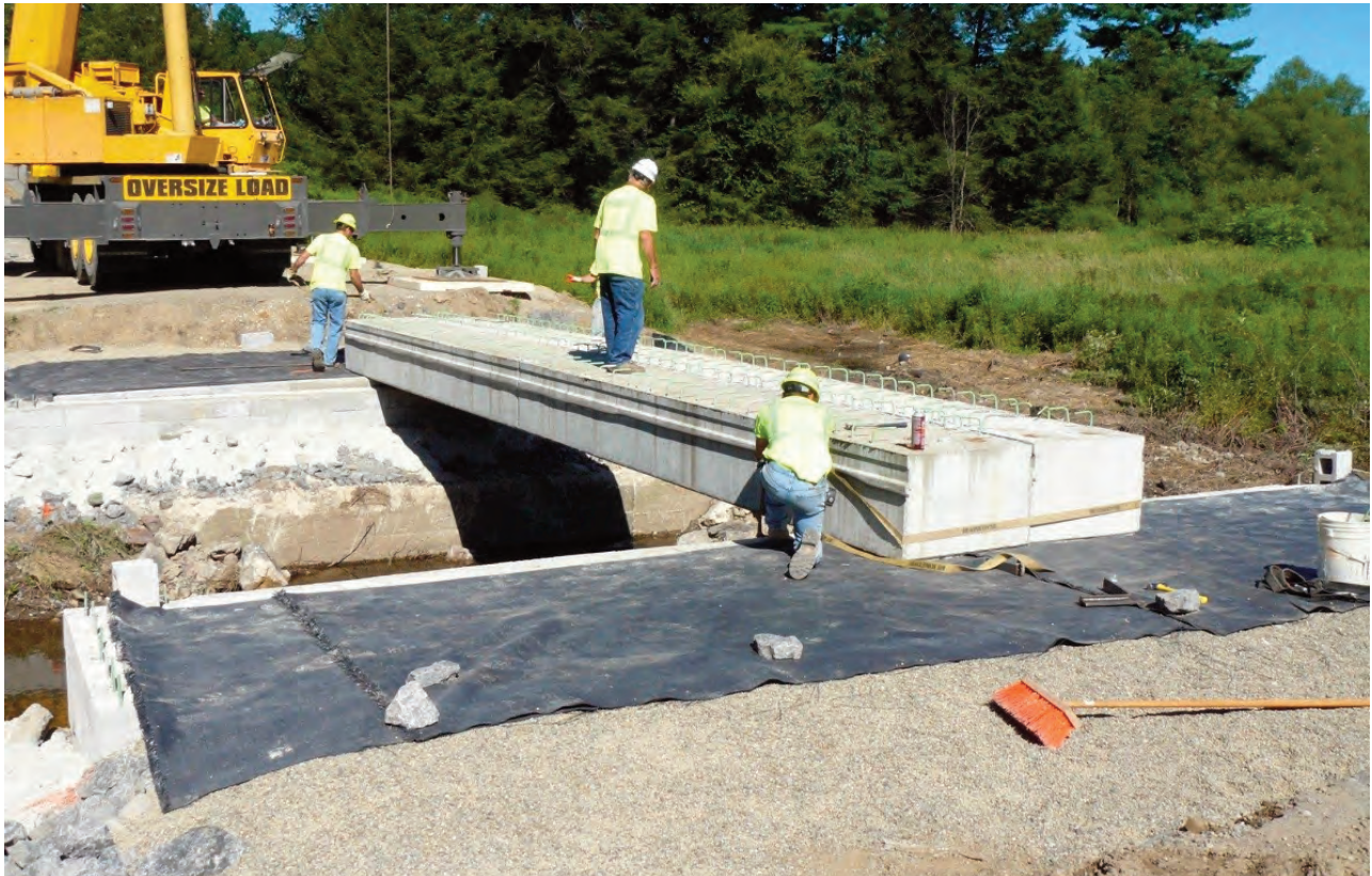
FIGURE 6. The Crawford County, Brown Hill Road (SR 1016) Bridge over Federal Run – Precast concrete channel beams for a concrete bridge deck installed on GRS abutments. District 1-0 accrued cost savings by fabricating the concrete channel beams in-house.
