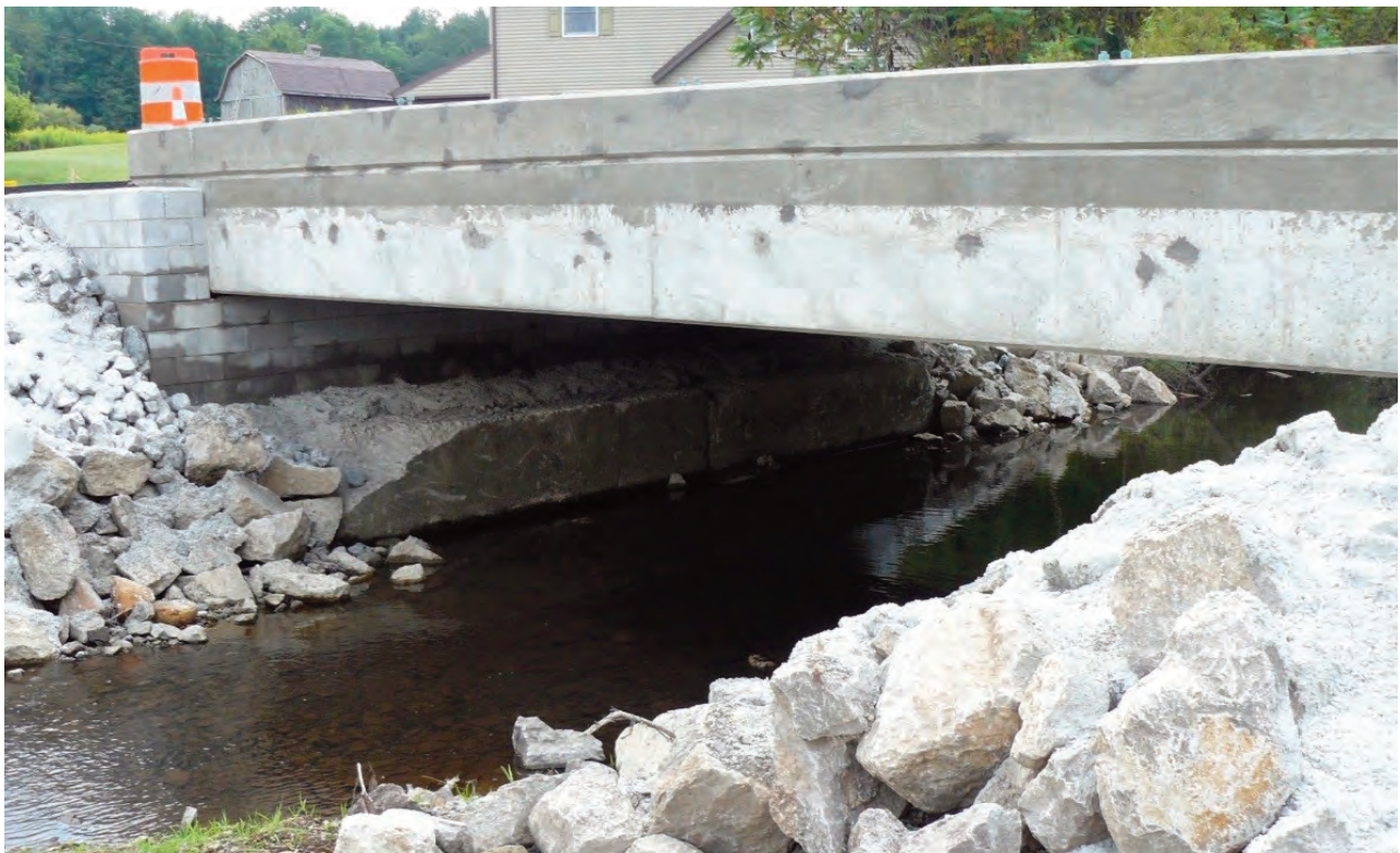
FIGURE 7. The Sandy Township, Clearfield County, Old Bliss Run Road Bridge over Mountain Run – Completed bridge.
