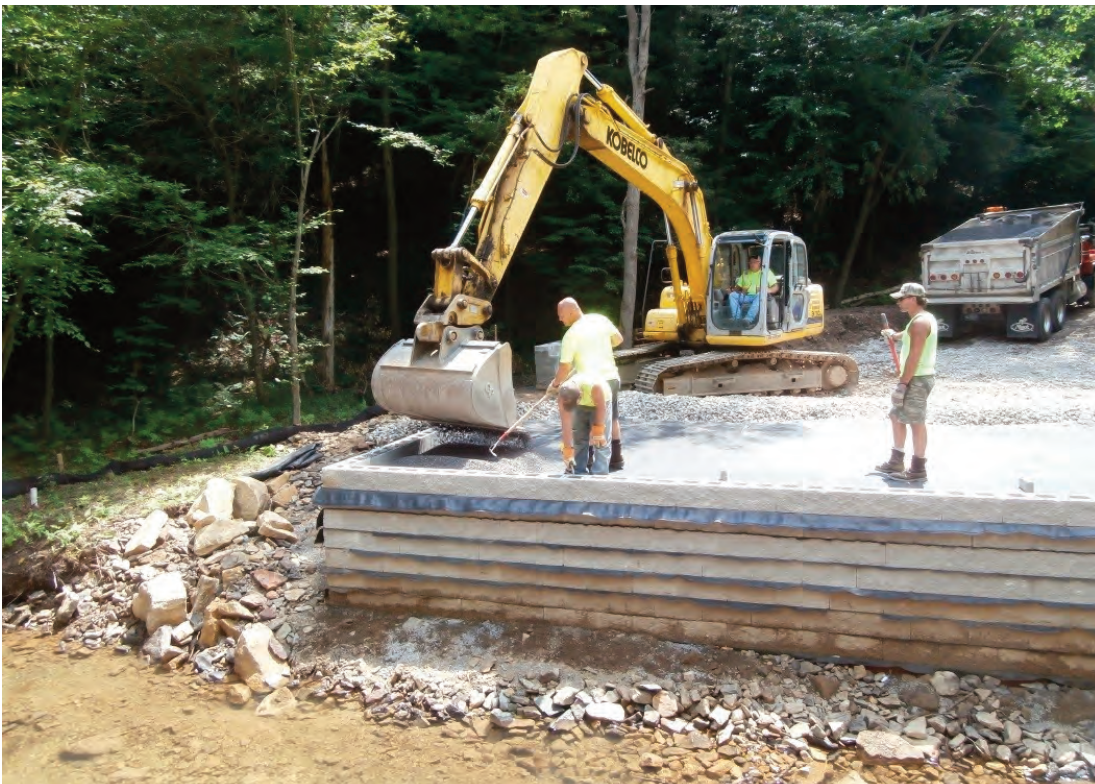
FIGURE 3. The Sandy Township, Clearfield County, Old Bliss Run Road Bridge over Mountain Run – Granular backfill placement.
