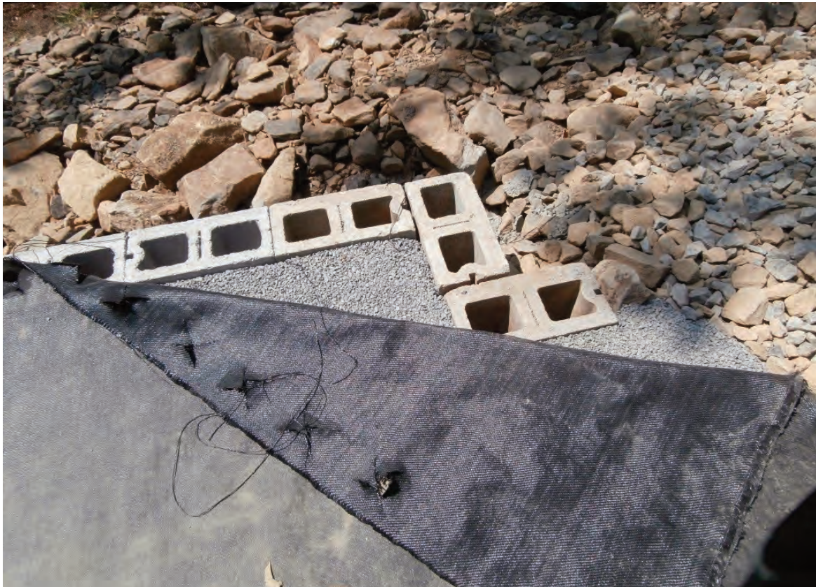
FIGURE 4. The Sandy Township, Clearfield County, Old Bliss Run Road Bridge over Mountain Run – Geosynthetic reinforcement, granular backfill, and CMU facing element. Note “X” cut in geotextile to allow for reinforcement/concrete placement.
