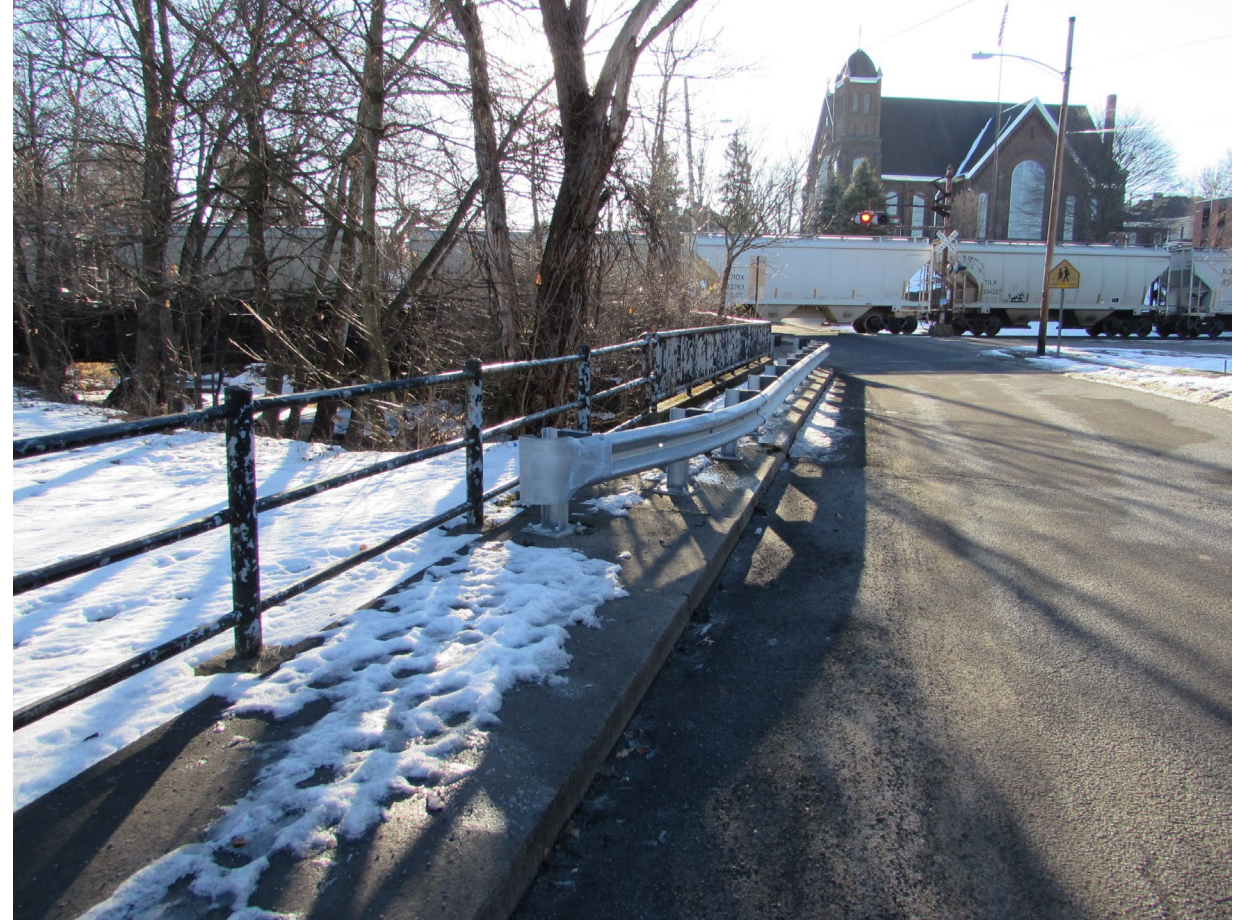
Closed Sidewalk On Bridge
