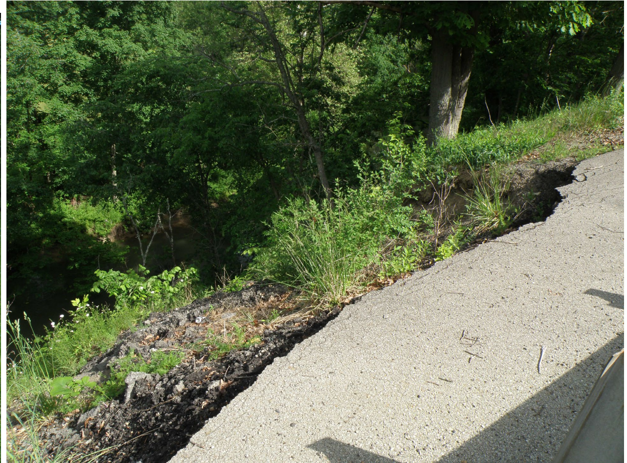
Slide Damage Behind Guiderail
