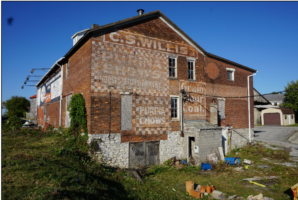
Photograph 7. East (side) and south (rear) elevations of the C. S. Willis Feed Mill, facing west.
