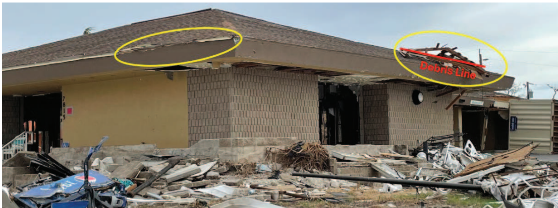
Figure 17: Rooftop Debris Line Example (Source: Cotality)
