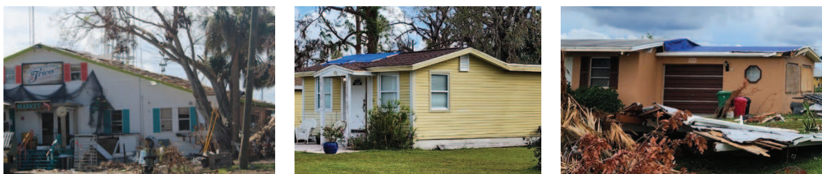
Figure 12: Wind Damage Examples (Source: Cotality)
