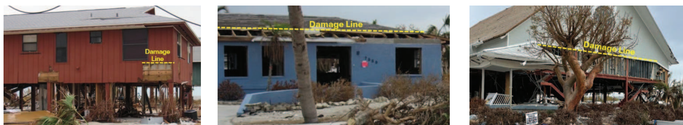
Figure 11: Damage Line Examples (Source: Cotality)
