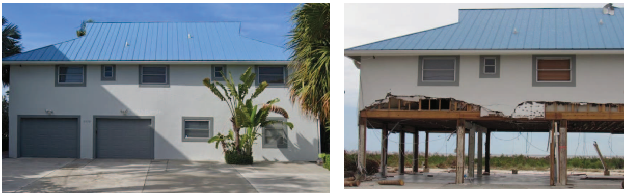
Figure 3: Example Before and After Flood Impacts on an Elevated Structure (Source: Cotality)
