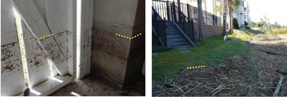
Figure 4: Example of HWM Evidence from Storm Events (Source: USGS)
