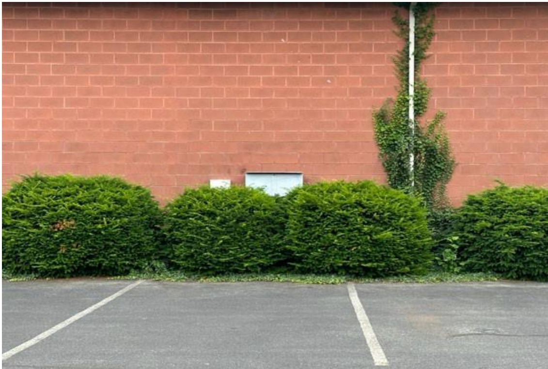
Main Electrical Disconnect North Side
