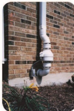
Typical fan and vent pipe.
