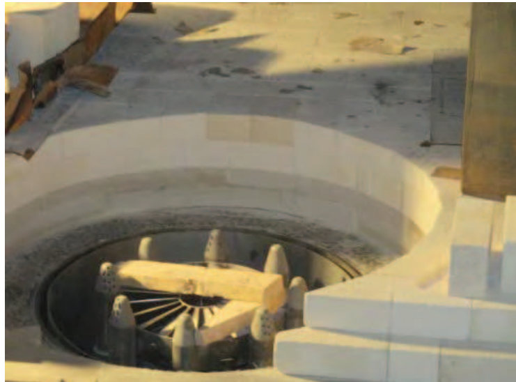
The stoker was removed and replaced with a floor built of plate steel and refractory. This image shows the vertically mounted burner and new floor.
