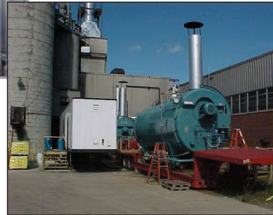
Installed Rental Boilers and Feedwater Trailer
