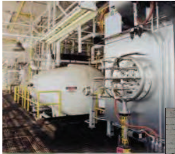
New Burner, Windbox and FD Fan along with a new Deaerator
