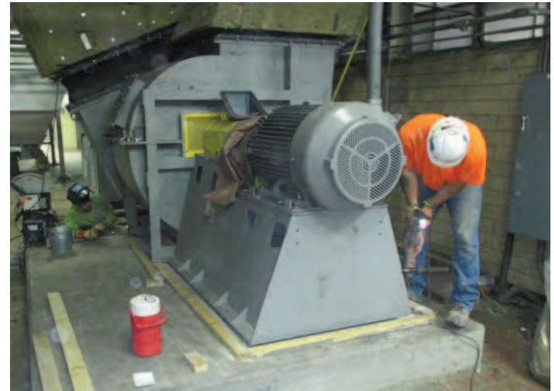
New fan for a converted boiler.
