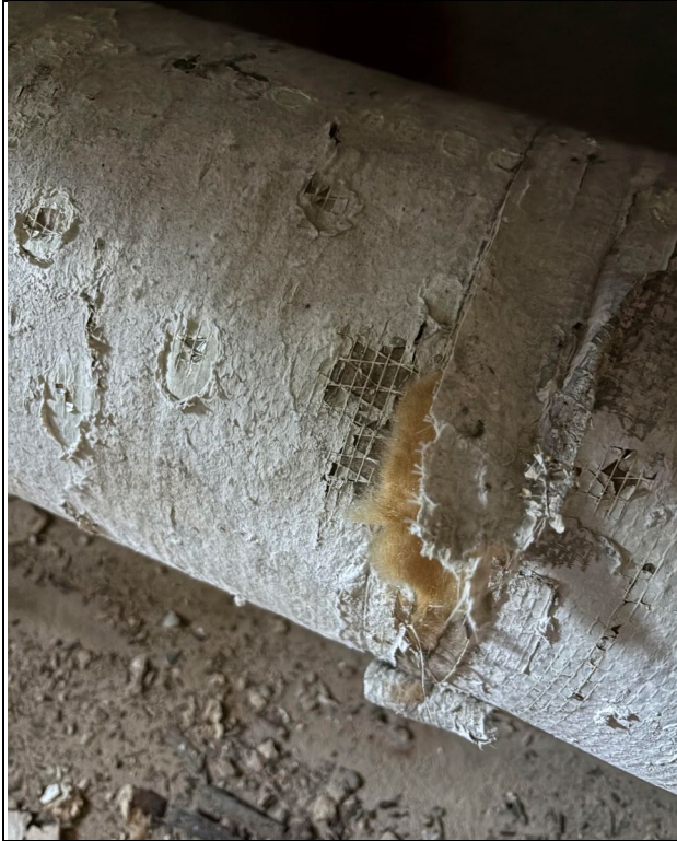
Photo 5 - HC-05A and HC-05B: White Paper Pipe Wrap and Yellow Insulation
