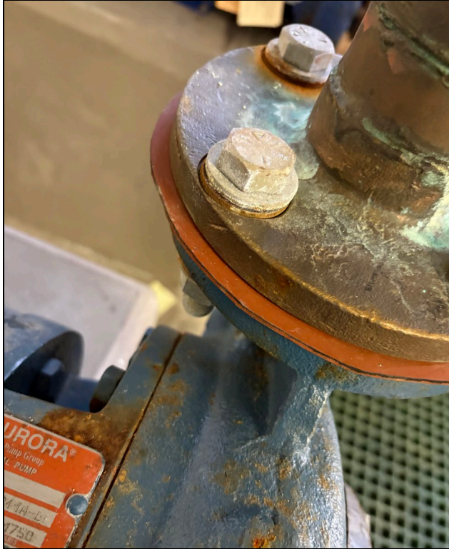
Photo 13 - HC-14 and HC-15: Red Pipe Gasket
