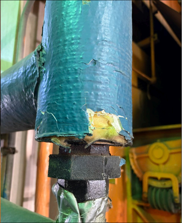
Photo 2 - HC-02A and HC-02B: White Paper Pipe Wrap and Yellow Insulation
