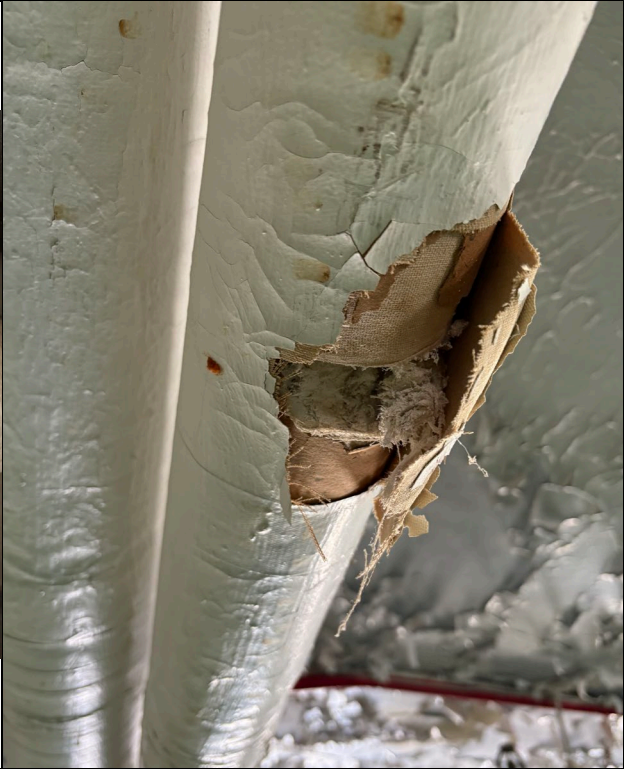
Photo 10 - HC-10: White Pipe Insulation – TSI (ASM)
