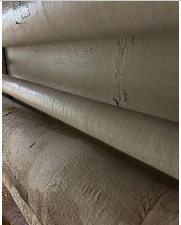
Photo 8 - HC-08: White Pipe Insulation – TSI (ACM)
