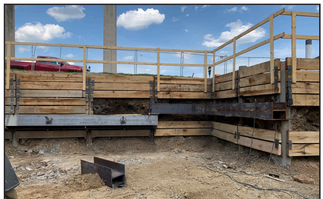
Progress of Shoring System Installed First set of Tie backs at Cooling tower Expansion
