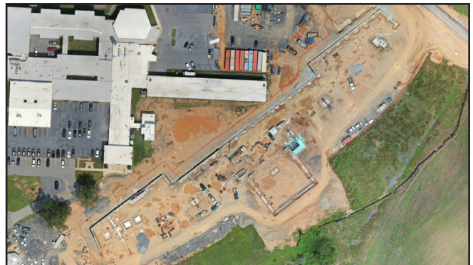
Overview of the Marquee Building footing and foundation layout within the project site
