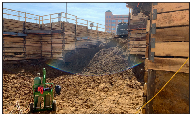
Progress of shoring System ready for second set of Tie back installation at Cooling tower Expansion
