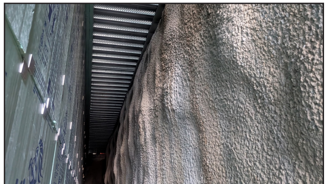
Depiction of the soil wall stabilization after the concrete foundation walls were installed
