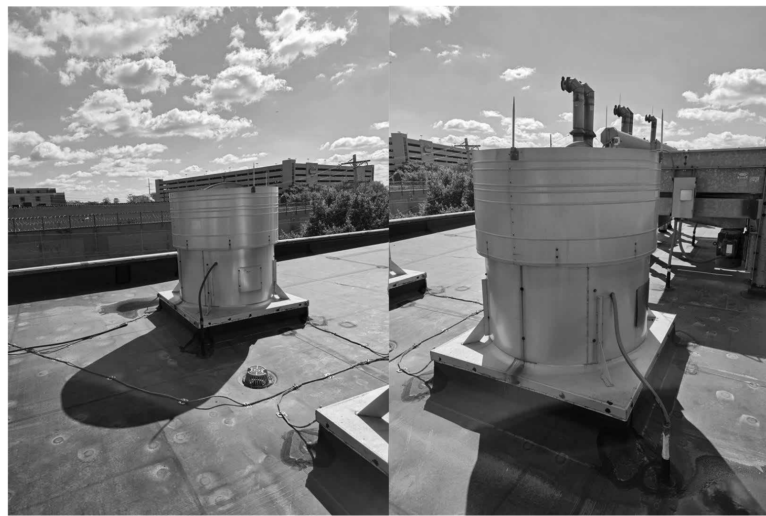
5 EXISTING ROOF EXHAUST FANS NOT TO SCALE
